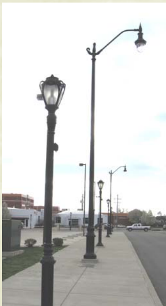
Downtown lighting similar to the historic lighting being installed on 5th & 6th St. in Enos Park
